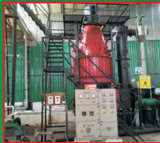
Producer Gas Unit
